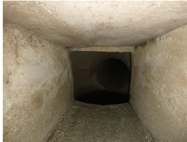
Exutoire pluvial (750x720mm)
