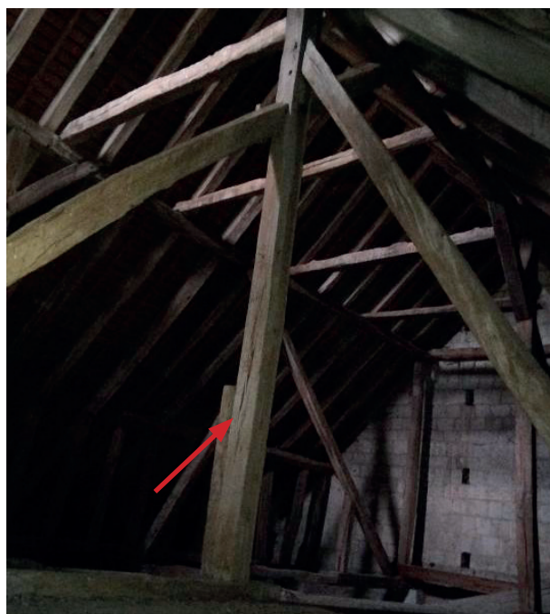
11. Poinçon gercé.(vaisseau principal de la nef).
