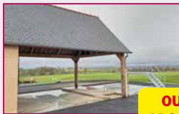
STATION DE LAVAGE
